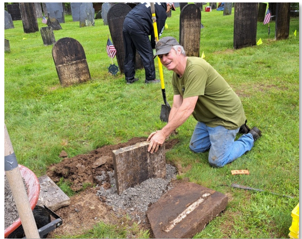
Chris Harlow straightens a crooked stoned and will use epoxy and clamps to repair the break.
